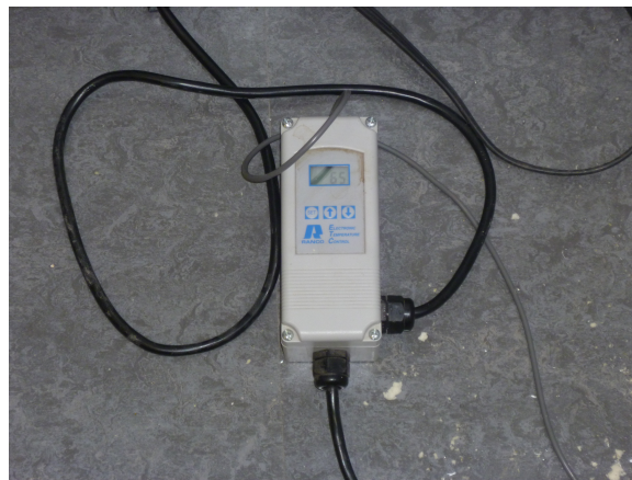
Figure A.4: Temperature controller used: Ranco Electronic Temperature Control.
